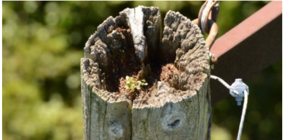
Pole top rot | Eversource
