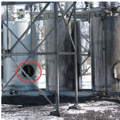
115-kV OCB catastrophic failure | Eversource
